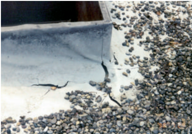
Figure 6.13: Lé d'étanchéité vieilli, photo GVL.
